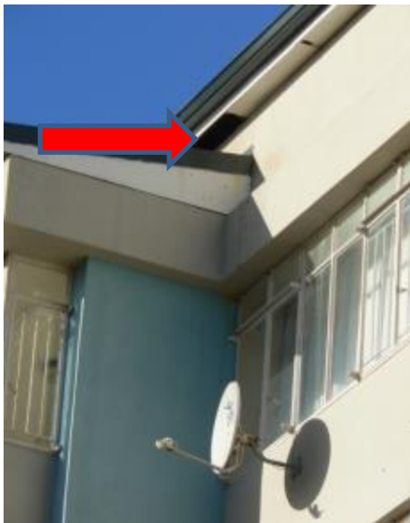
Figure 6: Hole in the eaves of the roof (see arrow) of the Bluefin flats that the baboons use to enter the roof and sleep there.
